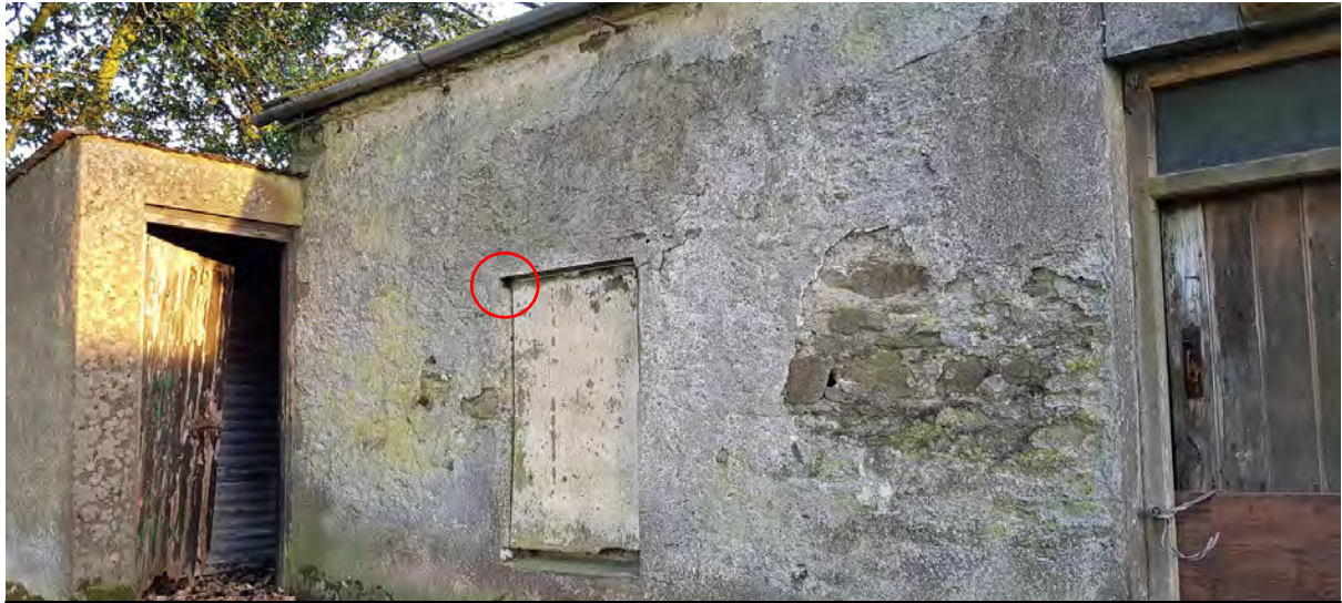
Photo 16 – Showing the emergence point, top-left corner of boarded-up window.
