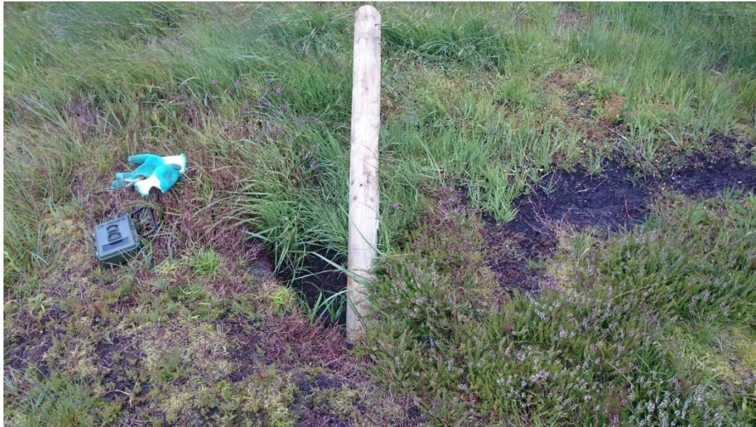
Plate 5 - The collapsed tunnel at 54745 11466 (bottom of post) with gloves and trail camera for scale.
