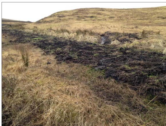
Plate 2 Main S-N drainage ditch cleaned out, with spoil spread to the side
