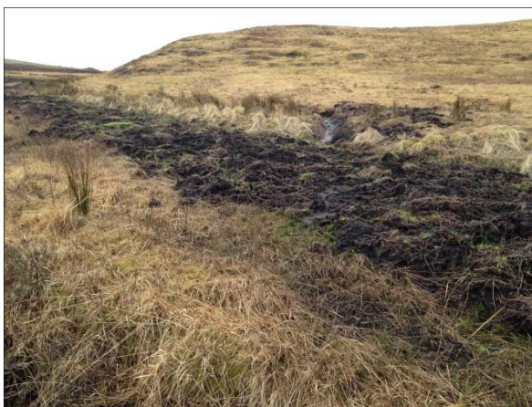
Plate 2 Main S-N drainage ditch cleaned out, with spoil spread to the side
