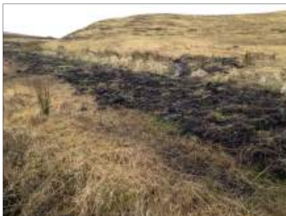
Plate 2 Main S-N drainage ditch cleaned out, with spoil spread to the side
